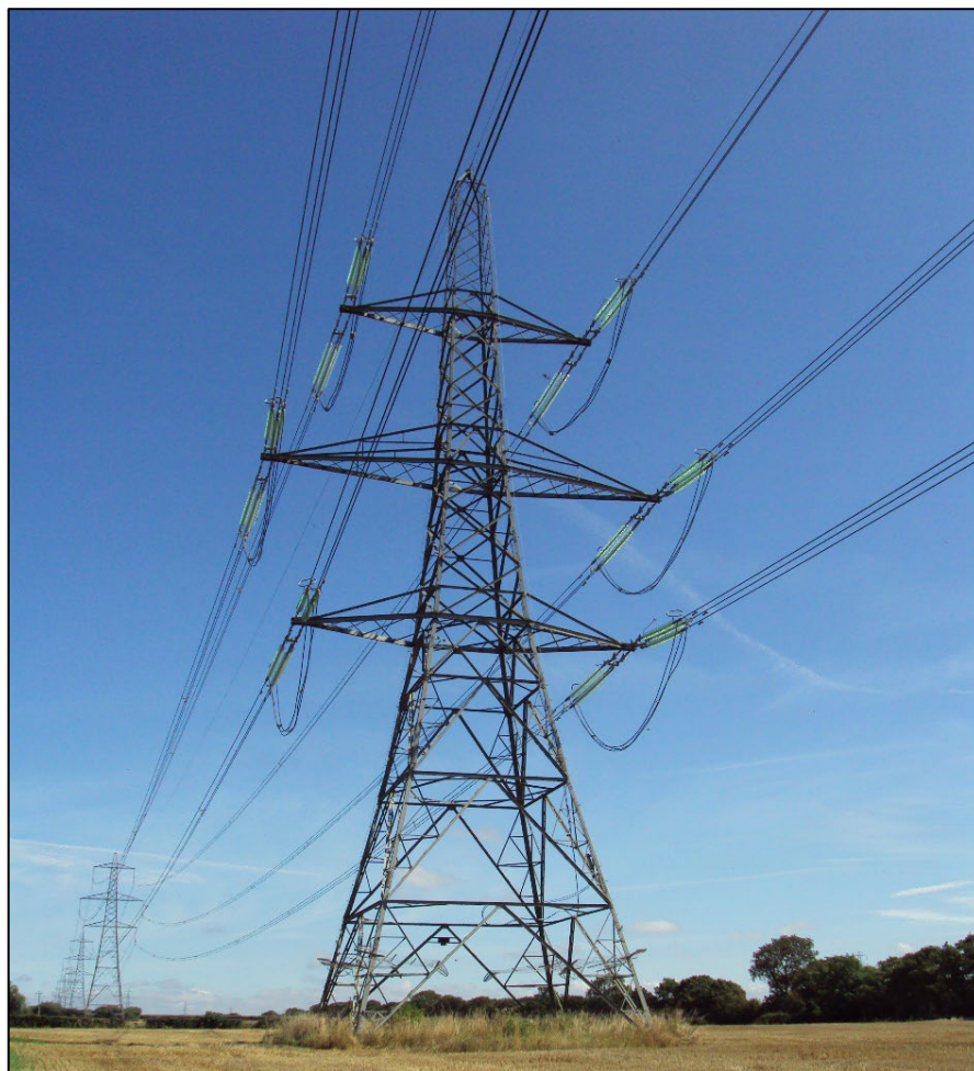
Figure 1 - 275kV Transmission Line
