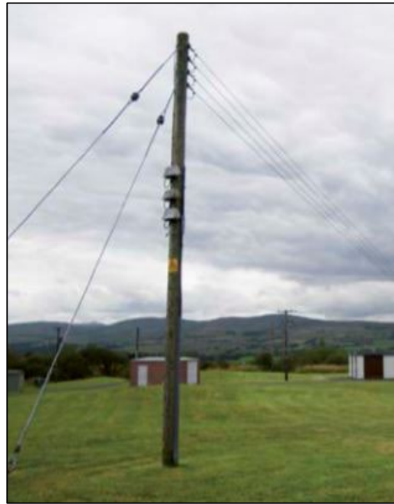
Figure 3 - 400V Distribution Line
