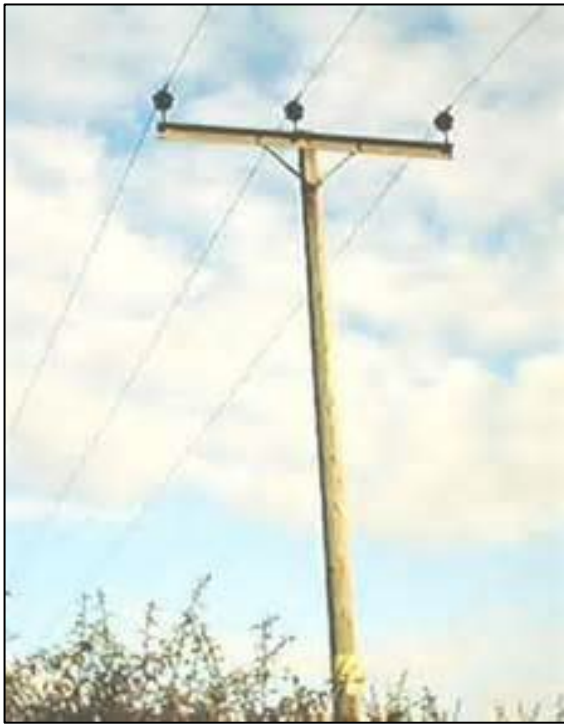
Figure 2 - 11kV Distribution Line
