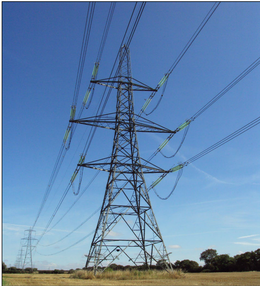
Figure 1 - 275kV Transmission Line
